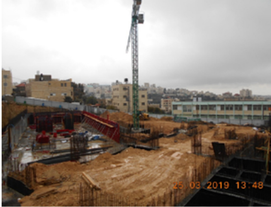
Tower crane erected and operational in block 1 and block 3 and part of block 2
